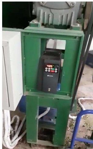
Gambar 3.24. Inverter 3 phase 5,5 kW
