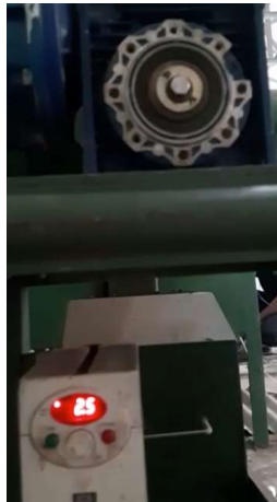
Gambar 3.25. Screw conveyor dan inverter
