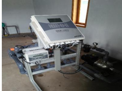
Gambar 11. Control panel NMC-PRO
